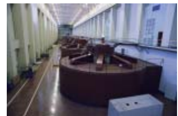
Mechanical equipment rooms
